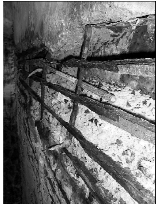
Exhibit IV. 3 Severely Deteriorated Reinforced Concrete
