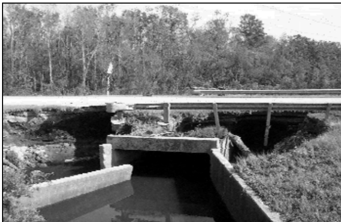
Exhibit IV. 2 Severe embankment erosion
