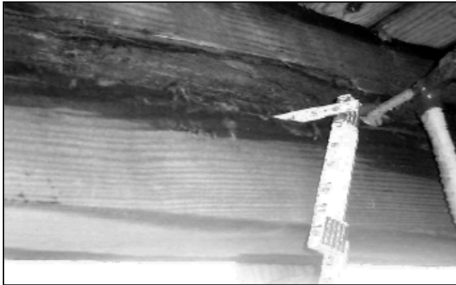
Exhibit IV. 1 Severely decayed timber beam
